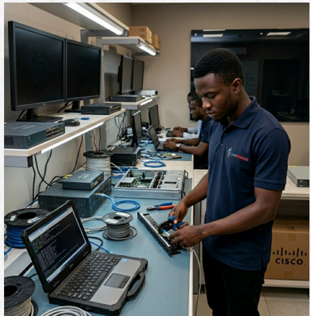
LAN Server room Set up project
