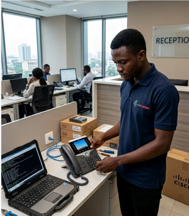
Cisco Unified Communication Installation project
